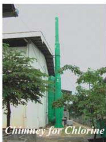
Scrubber for Chlorine
