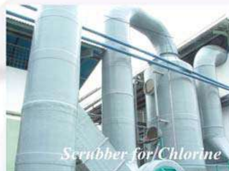
Ducting for Gas Chlorine
