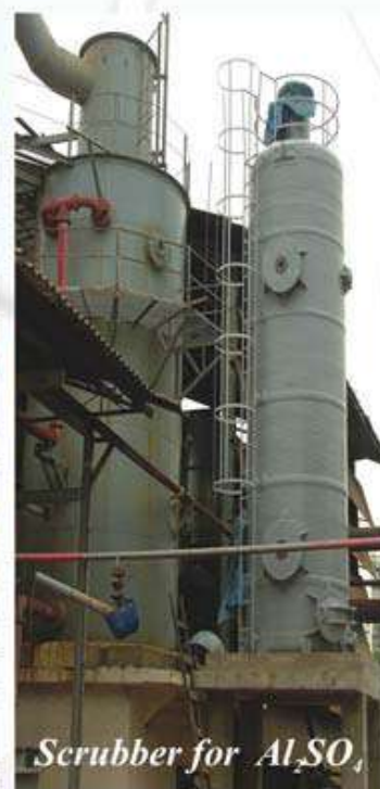
Co. Purification System
